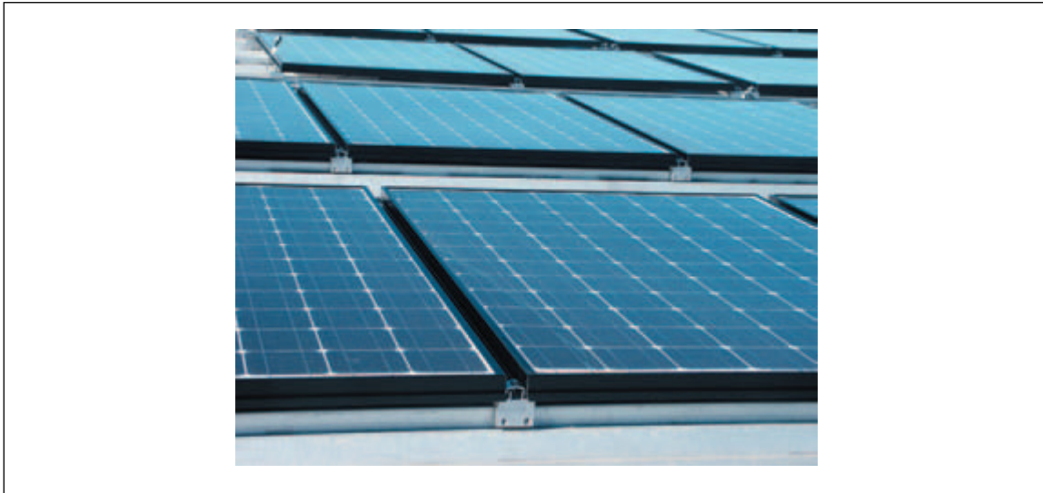
Fig. 3.2.2a. Solar panels secured to standing seam roofs using external seam clamps
