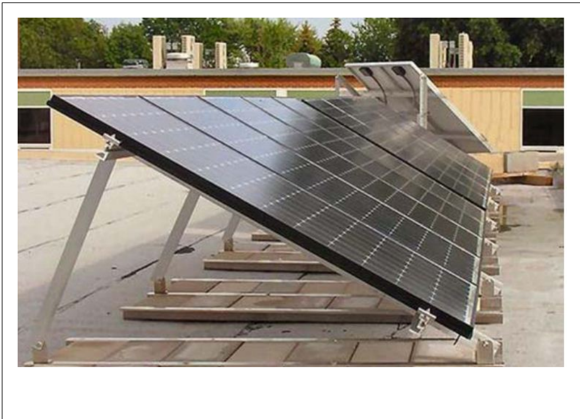
Fig. 3.2.1.1b. Solar panels with steeper slopes or lacking wind deflectors will experience greater wind effects
