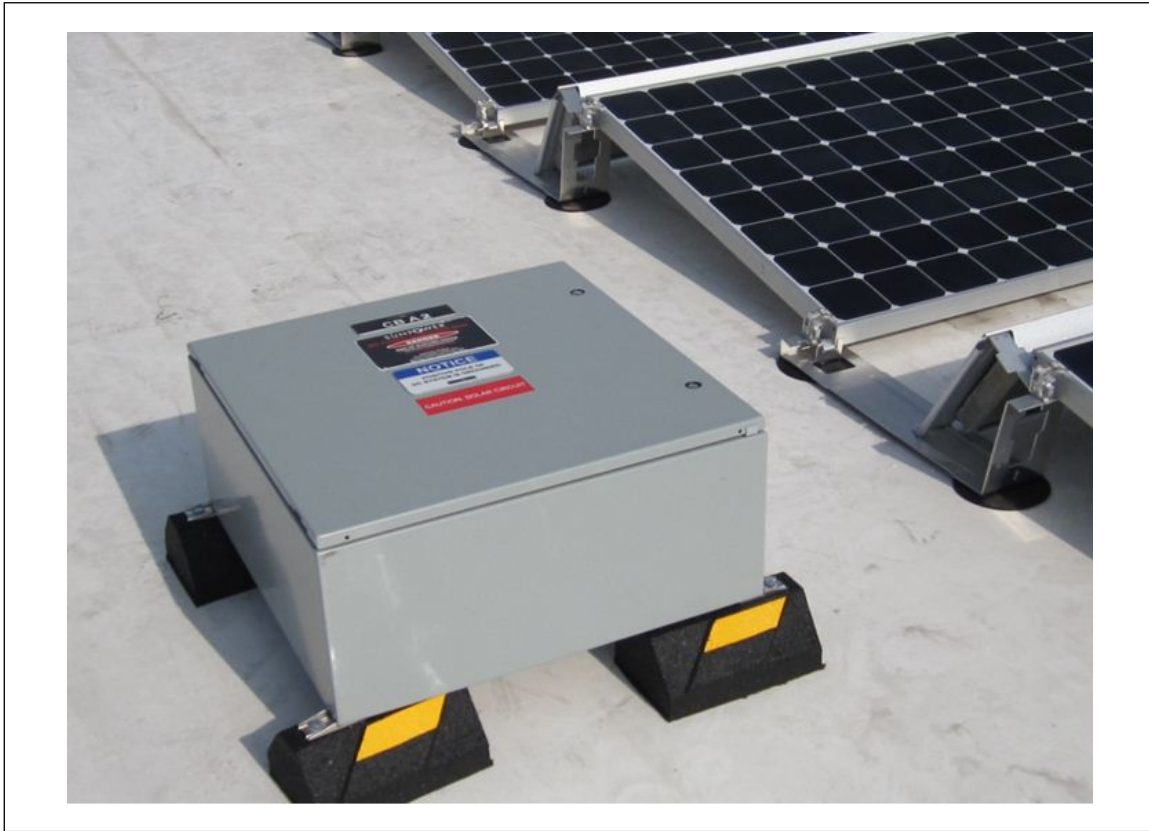
Fig. 3.2.1.1c. Equipment lacking anchorage to roof framing
