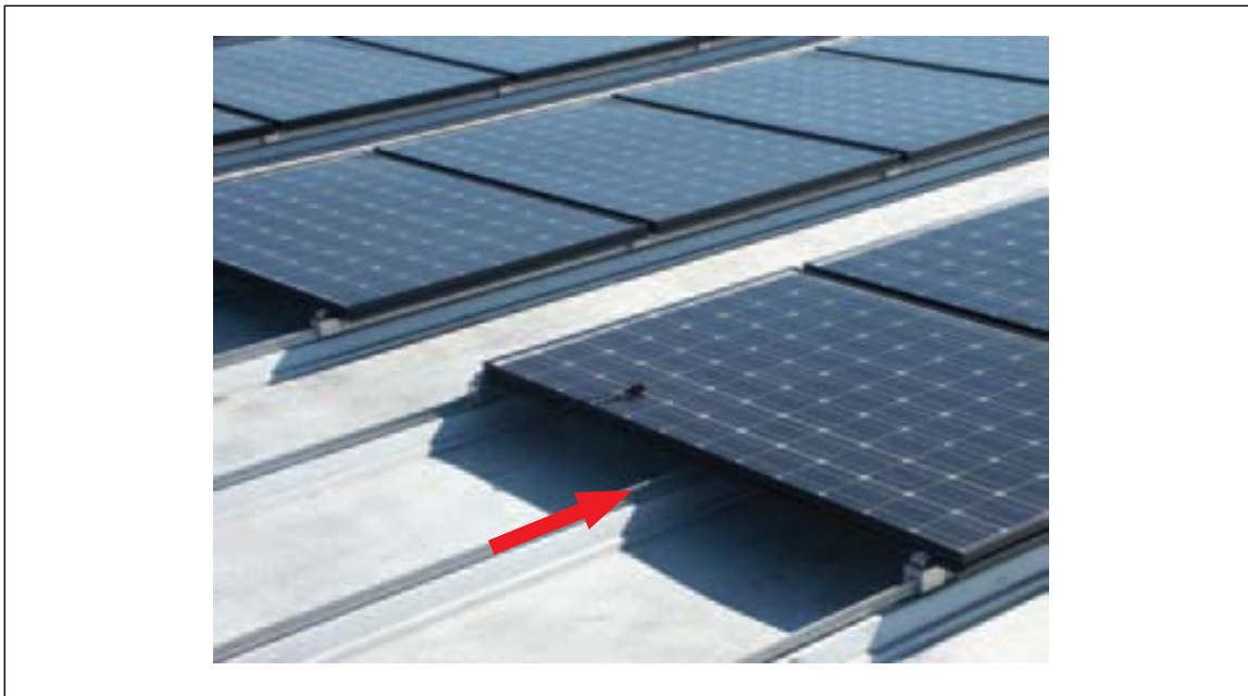
Fig. 3.2.2b. Unacceptable arrangement unless specifically tested and FM Approved: clamp missing from SSR rib below middle of outer panel edge
