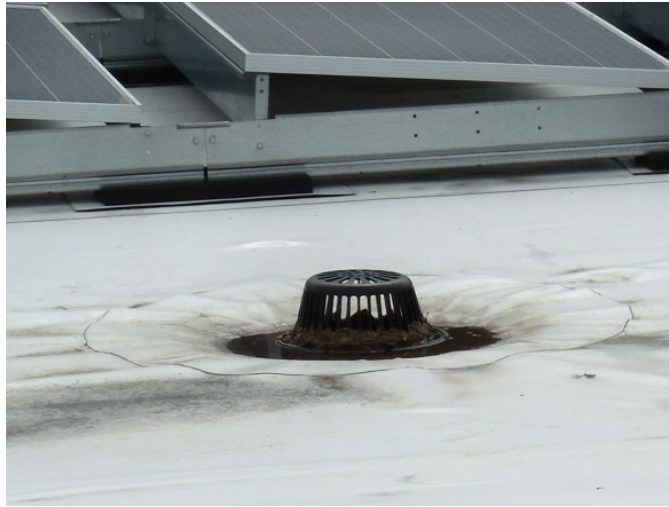
An example of a roof drain on a low-slope roof adjacent to PV modules. (Source: ZRS)
