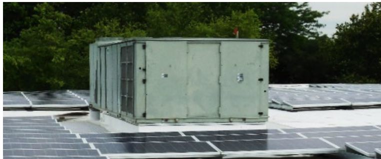
An example of a large piece of rooftop equipment adjacent to PV modules. (Source: ZRS)
