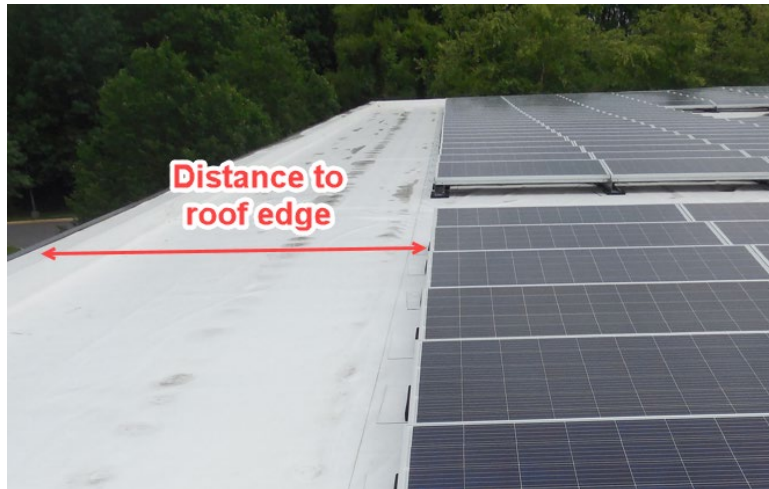
An example of a PV system roof edge setback. (Source: ZRS)
